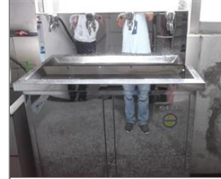
Photo of the sanitary facilities Drinkable water.JPG
