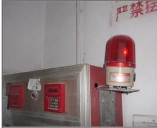
Photo of fire safety equipment Fire alarm.JPG
