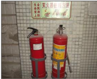
Photo of fire safety equipment Fire extinguisher.JPG
