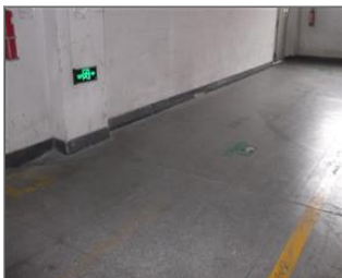
Photo of fire safety equipment Evacuation directional sign.JPG
