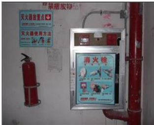
Photo of fire safety equipment Fire hydrant.JPG
